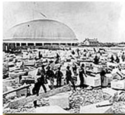
Granite blocks to be used in the construction of the temple. Tabernacle and Endowment House can be seen in background.
